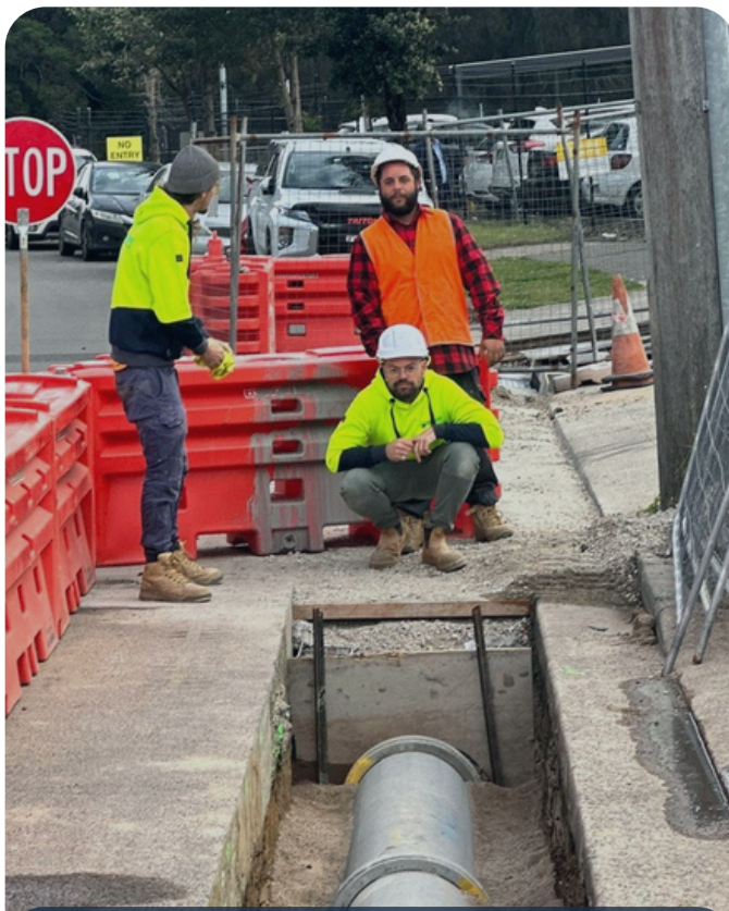
In-ground stormwater — 6C The Crescent
