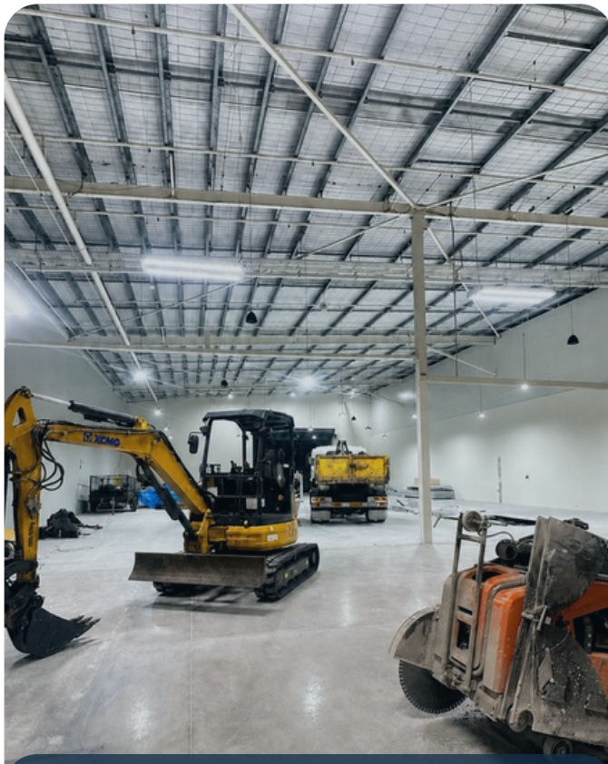
Inground Hydraulic Services
